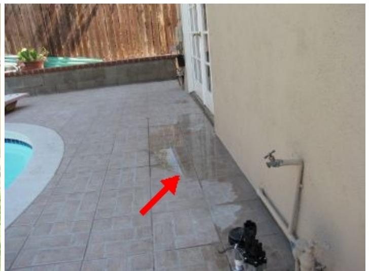
Pool deck is sloped toward house where water collects
