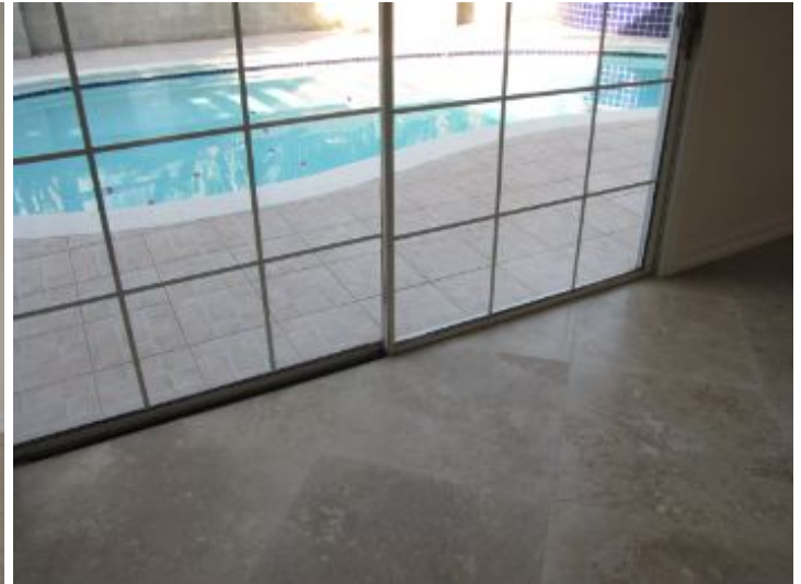
Sliding glass patio doors do not slide well and are difficult to open
