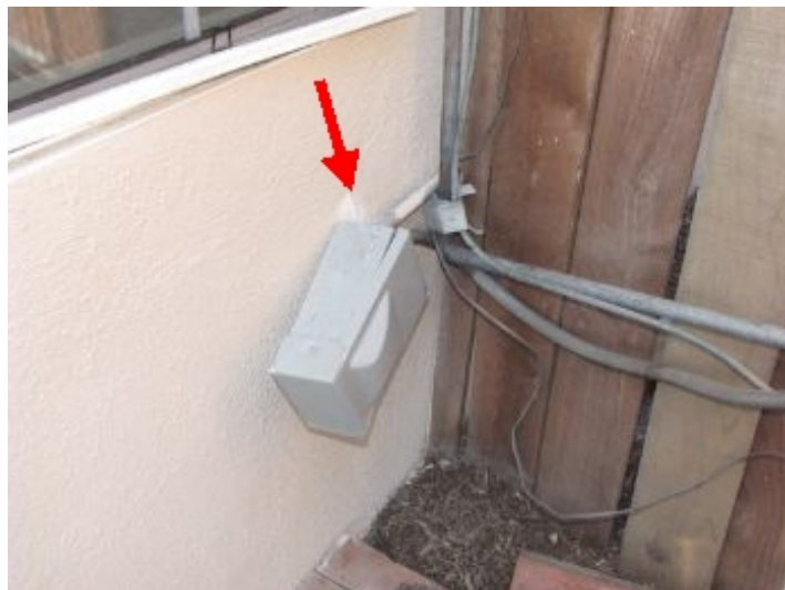
Shutoff switch to AC condenser not secured
