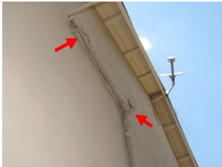
Insulation on Refrigerant lines is deteriorated
