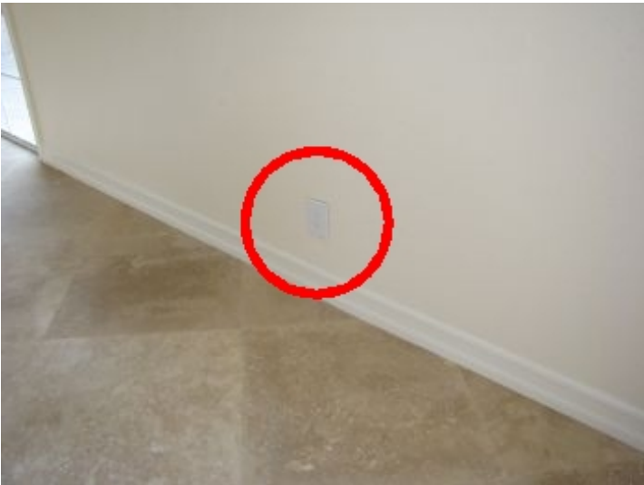
Loose electrical box in kitchen wall
