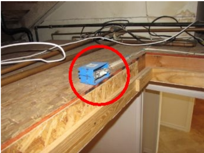
Missing cover plate at light switch box in attic
