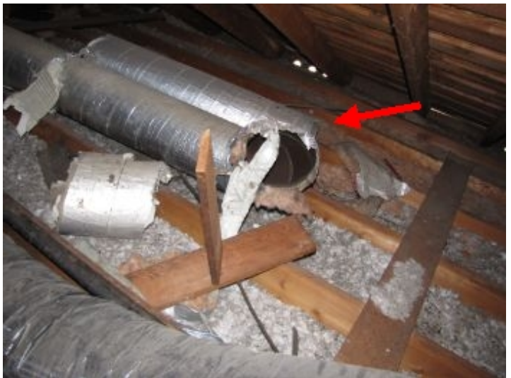
Discarded ducting in attic
