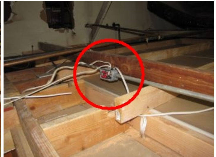
Cover plate missing at junction box in attic
