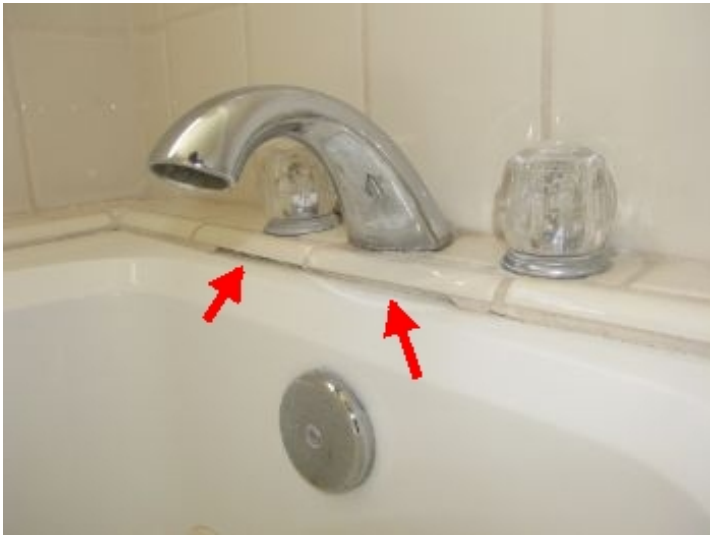
Spalling grout at 2nd floor bath tub rim
