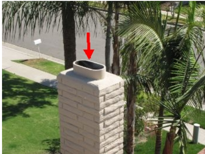
Spark arrestor not present at chimney
