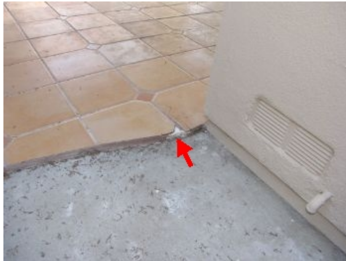
Deteriorated deck tile at rear patio area
