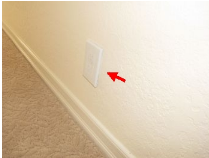
Loose electrical boxes in bedrooms
