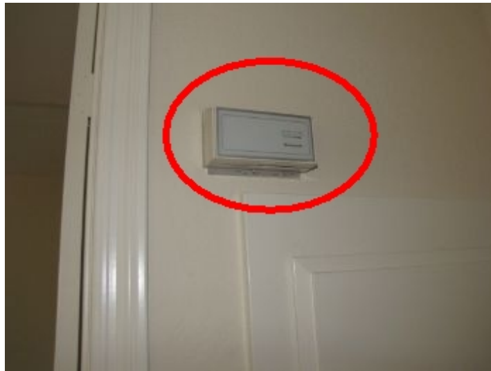
HVAC did not respond to thermostat, recommend evaluation by HVAC technician
