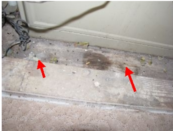
Rodent droppings in furnace closet
