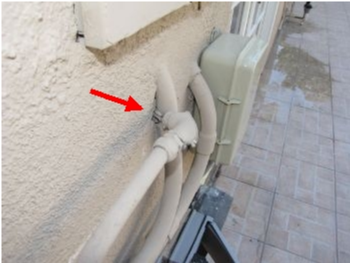
Conduit servicing pool equipment is broken
