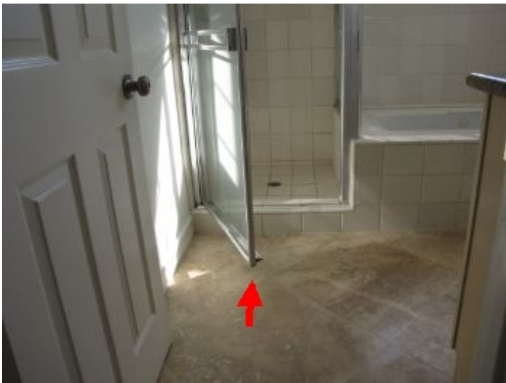
Shower door sweep at 2nd floor bathroom is deteriorated
