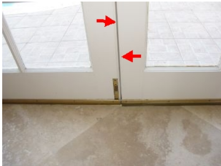
Daylight shows through weather stripping
