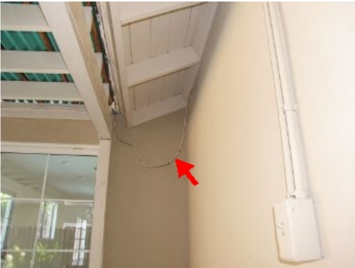
Unsecured cable wire at patio eave
