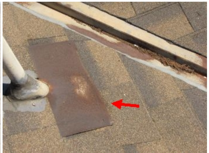
Suggest painting of vent flashing to control rust scale (flashing is in satisfactory condition)
