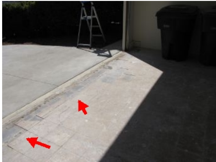
Loose & missing vinyl floor tiles in garage
