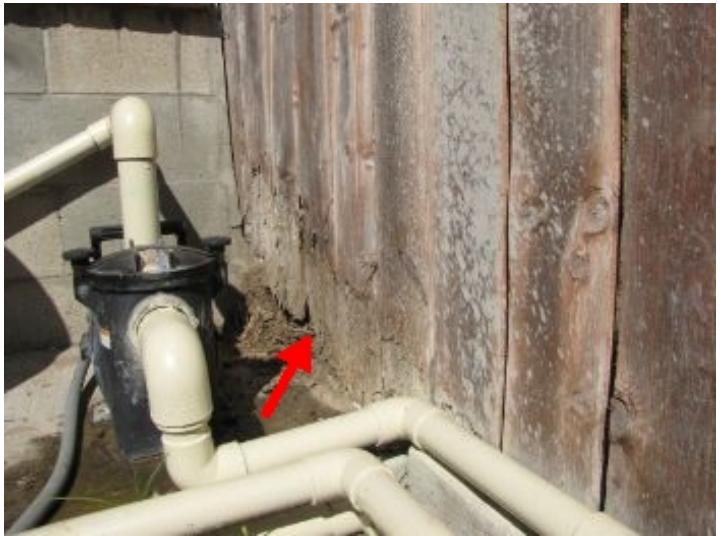
Deterioration of fence boards at pool pump
