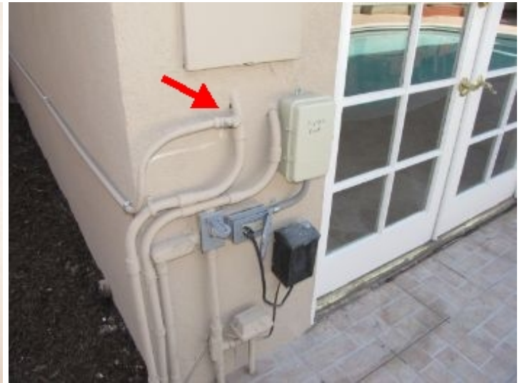
Area where conduit servicing pool equipment is broken
