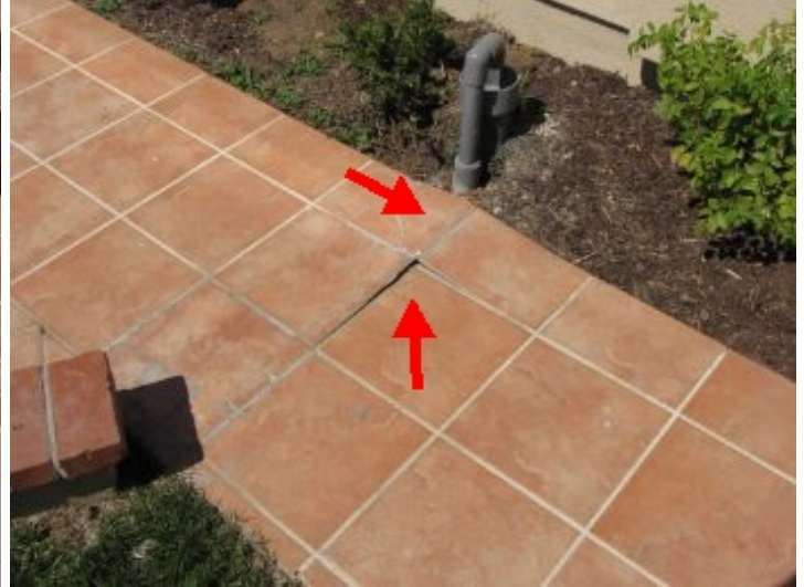
Loose tiles at walkway planter
