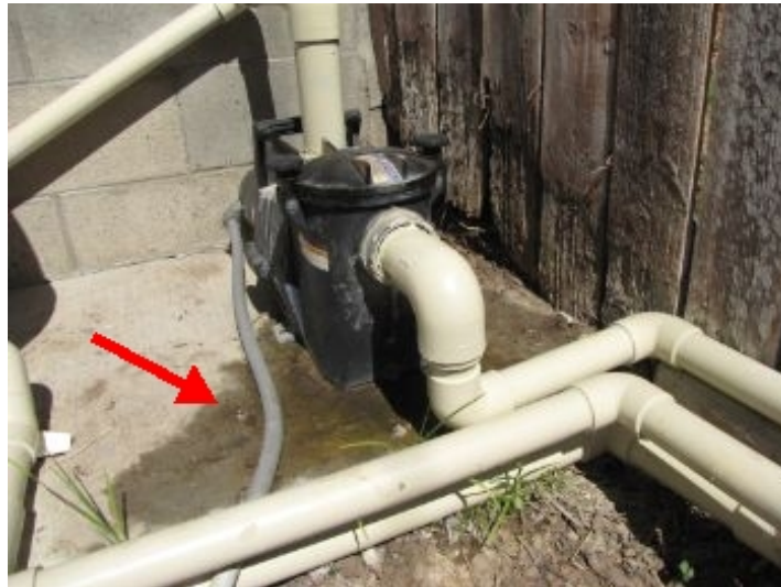
Pool pump has a water leak
