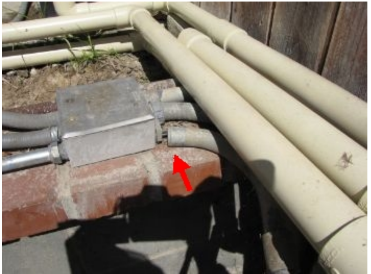
Electrical conduit at pool equipment has a broken conduit connection
