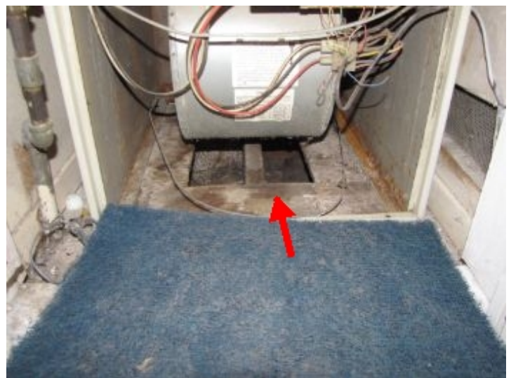
Holes cut for air passage appear small, recommend evaluation by HVAC technician
