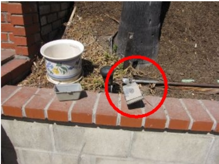
Outdoor electric functions correctly but is not secured
