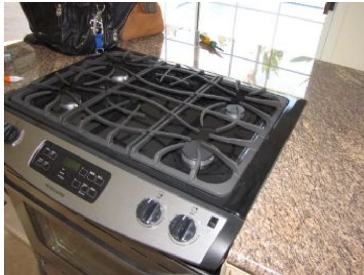
Kitchen stove does not appear to have venting (no hood above or downdraft below)
