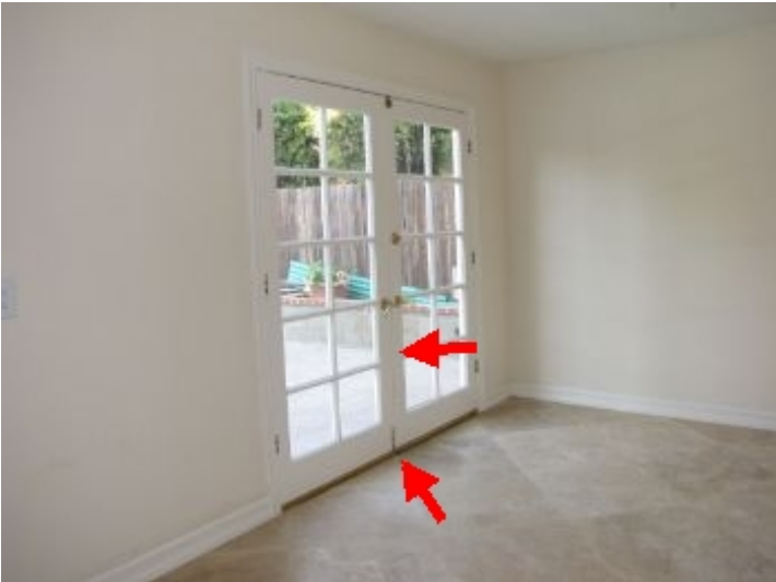
French doors at patio do not shut securely and weather stripping shows daylight
