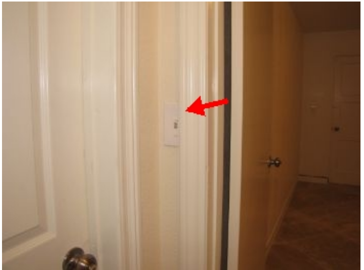
Light switch for laundry room is buried under molding in hallway
