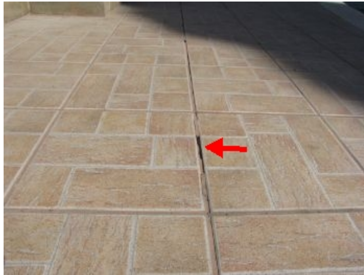
Spalling grout at pool deck
