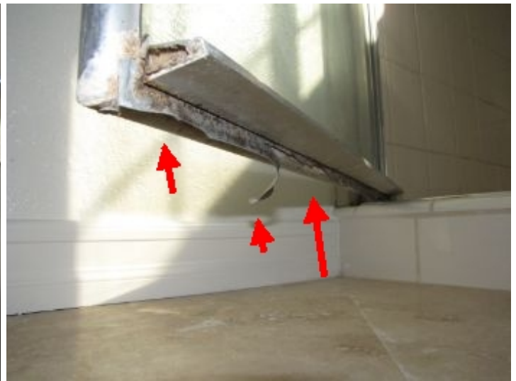
Deteriorated shower door sweep at 2nd floor bathroom
