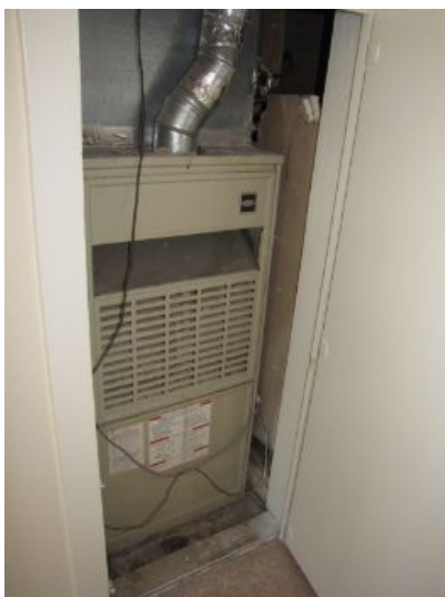
View of furnace/closet
