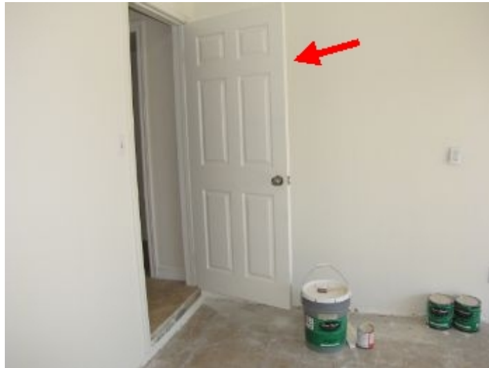
Non fire rated door to garage to interior
