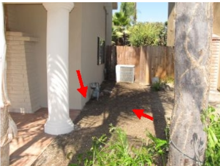
Soil at right side of house is not sloped away from foundation
