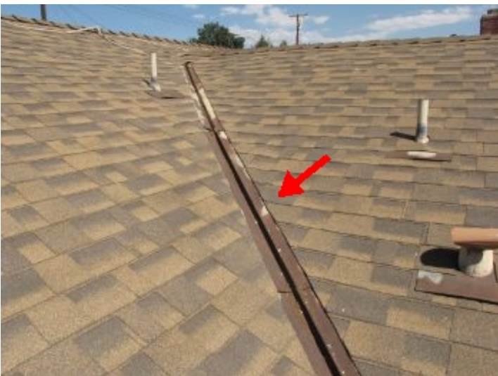
Suggest painting of valley flashing at roof to control rust scale (flashing is in satisfactory condition)
