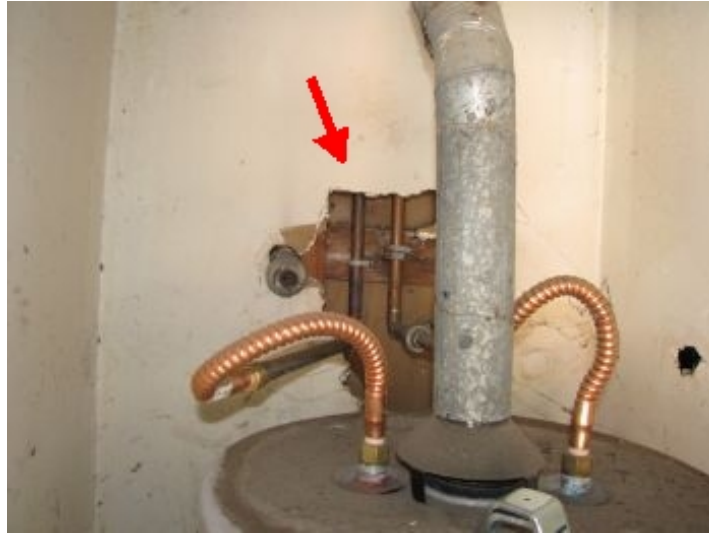
Un-patched wall in water heater closet
