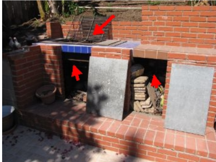
Outdoor grille is plumbed for gas but is not operable
