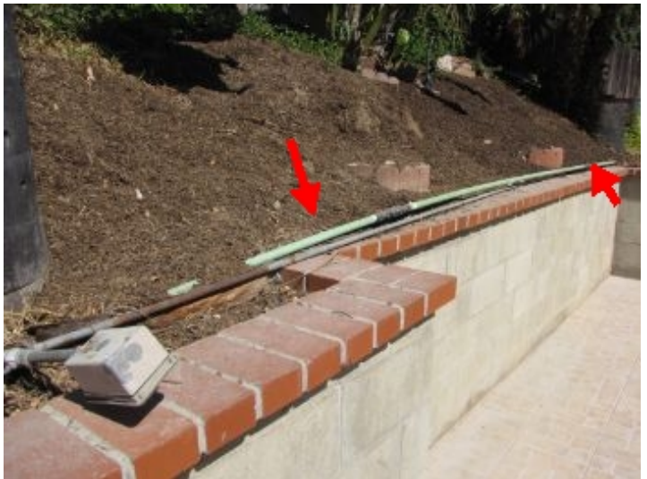
Gas line to pool equipment and Bar-B-Q is not buried the required 12-18"
