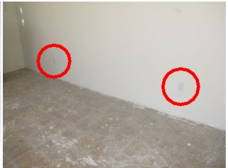
No power to two electrical outlets in garage (wall backs to laundry room)
