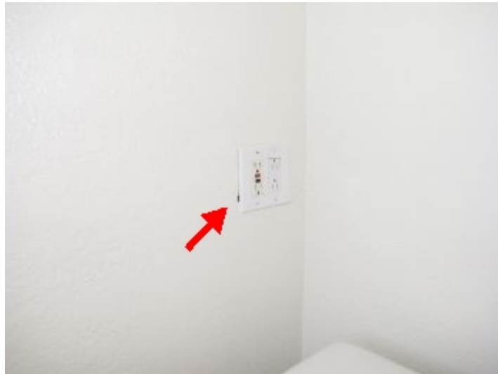
Void at wall switch in 2nd floor bathroom
