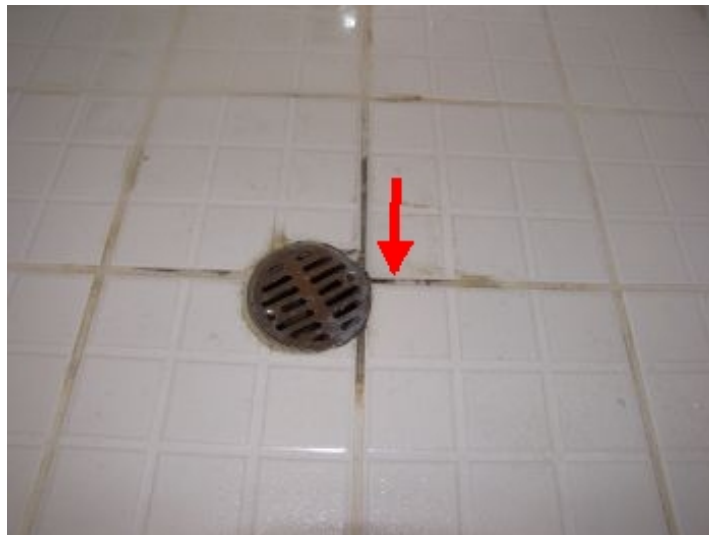
Spalled grout in 1st floor bathroom shower pan
