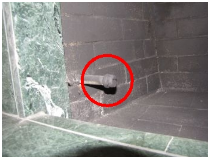
Gas service to fireplace is capped off and functionality not verified
