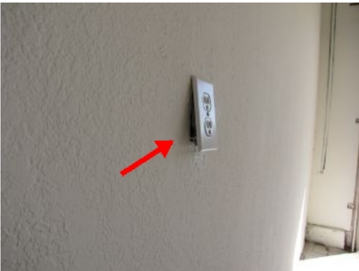
Loose electrical box in garage
