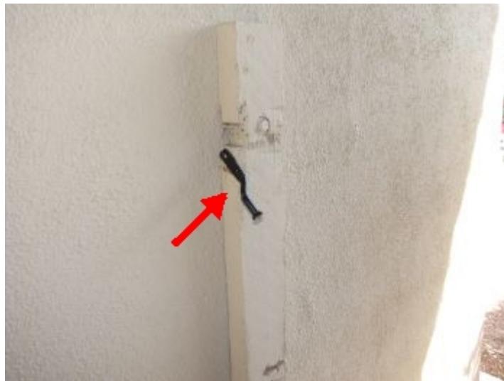
Gate latch needs adjustment
