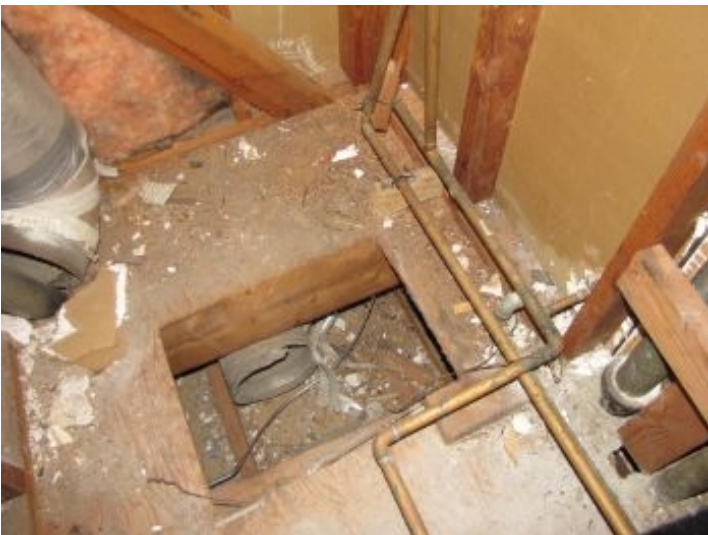
Debris and discarded ducting left in attic
