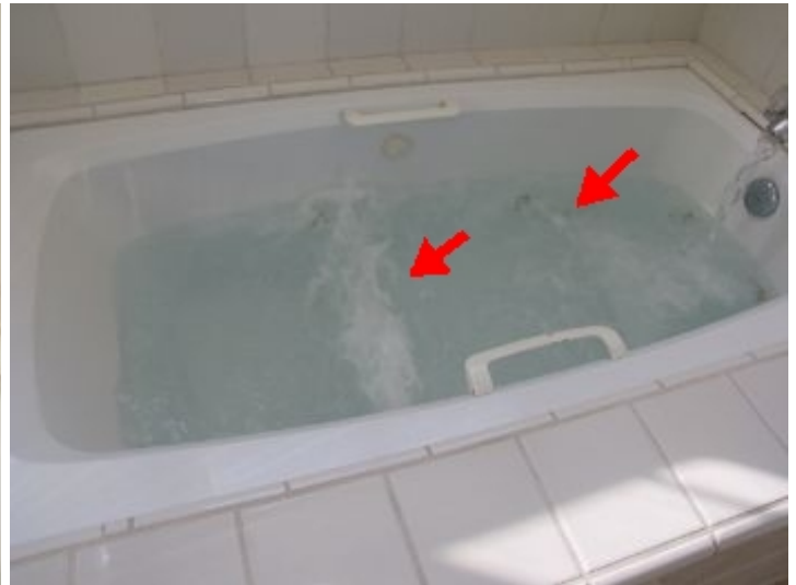
Jets function well at 2nd floor bath tub
