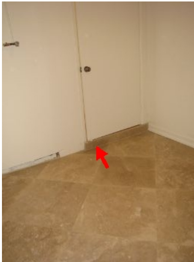
Door to laundry drags on floor and difficult to open/close
