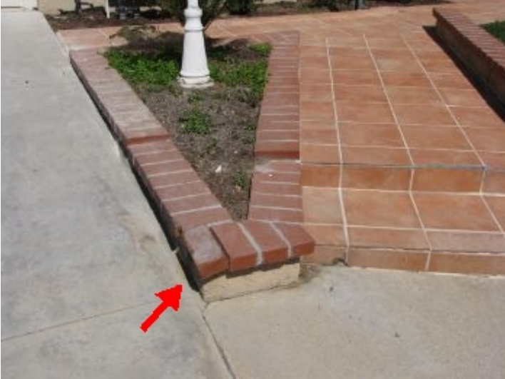
Loose bricks at walkway planter
