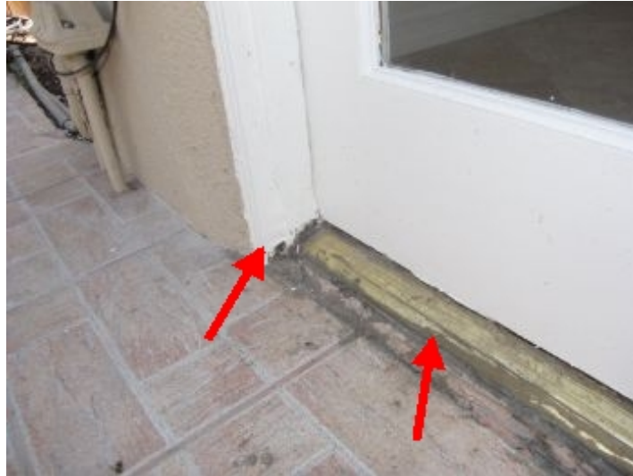
French doors affected by improper pool deck drainage
