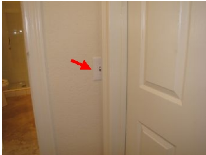
Light switch in hallway buried under molding
