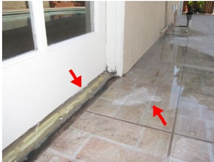
Water from pool collects at door threshold, suggest grate drain be installed
