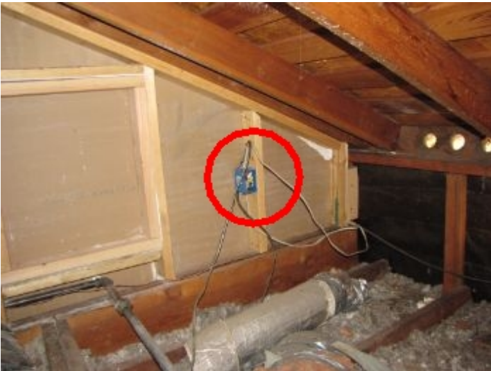
Missing cover plate and loose wires in attic
